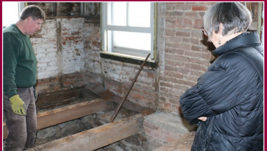
Adam Wengryn, of Restoration Technologies, and Catherine Suttle, HLT's Director of Cultural Resources, discuss the reconstruction of the back entrance to the Dvoor Farm House.
